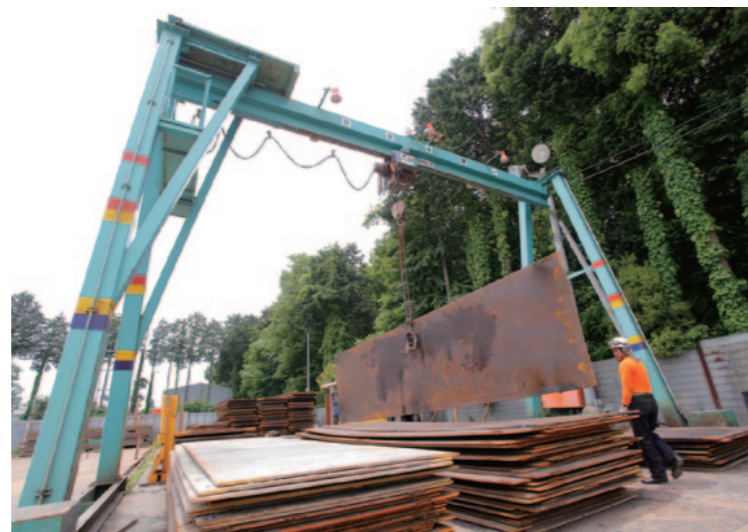
Steel plates from Hanwa Eco Steel Corporation are being used in a variety of sites, including rentals for use as scaffolding in road repair in disaster areas
